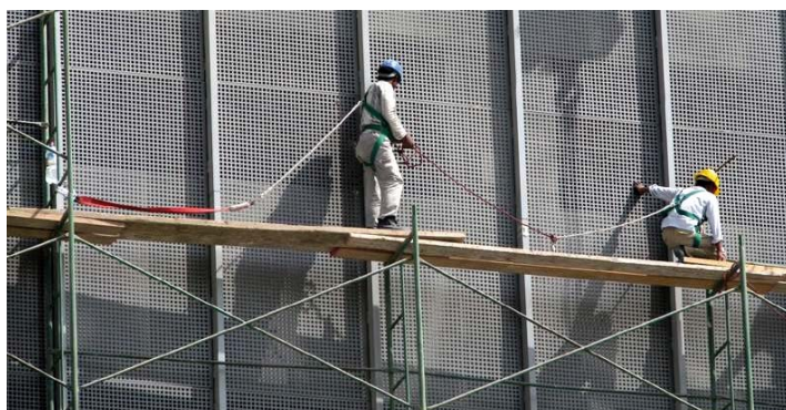
Engineers tried to follow international safety practice but failed as evidenced by the workers wearing harnesses, but doing so dangerously.
