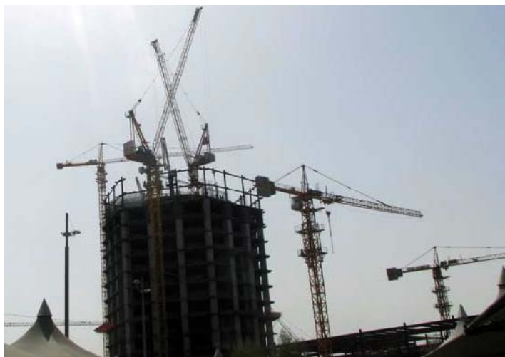
The Doha skyline as the city into the desert. The cranes swing 24 hours a day to meet building deadlines.
